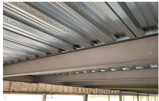
Overlapping Joint at bottom of I-Beam
