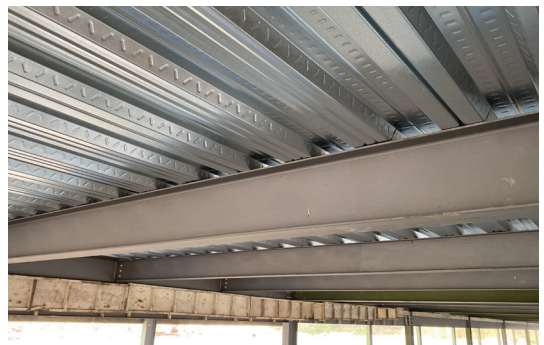
Overlapping Joint at bottom of I-Beam
